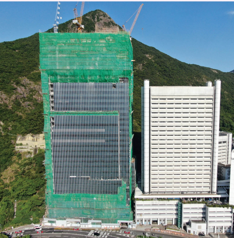
施工中的臨床大樓1於街道視角 Street view of Clinical Block 1 under construction
